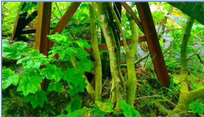
PHOTO 3: Vegetation growing in and around supports
