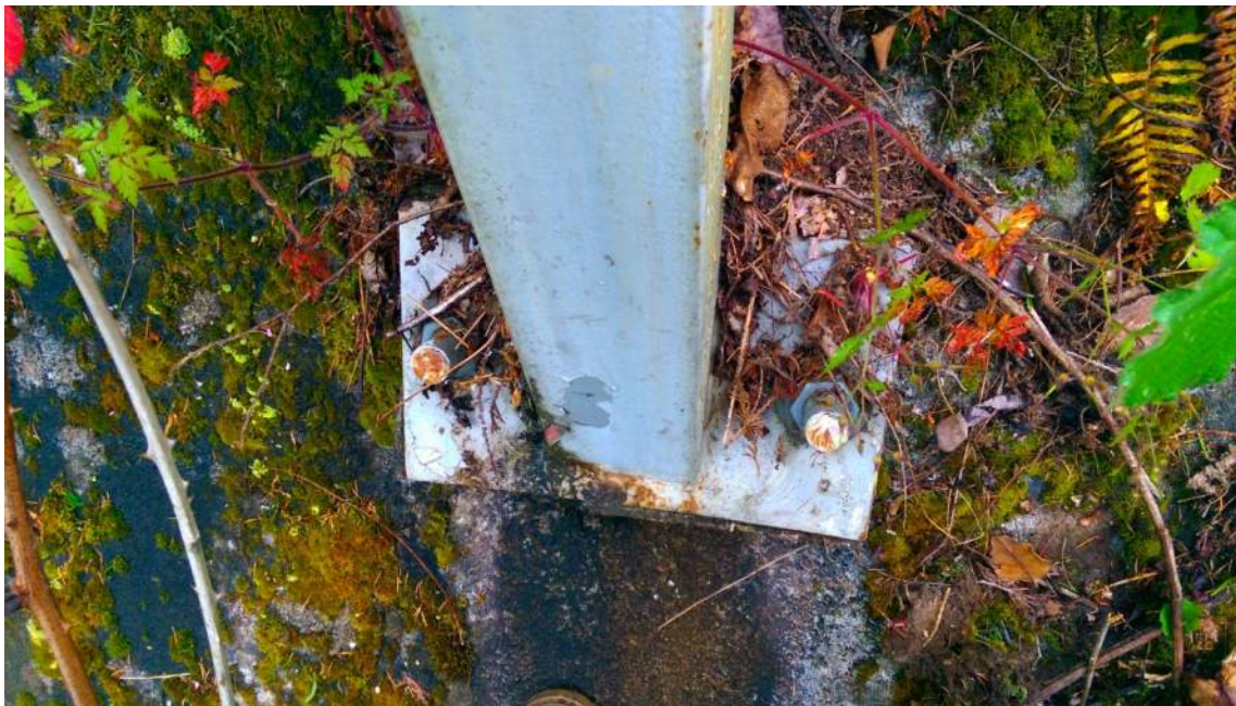
Photograph 6 Baseplates buried in organic matter.
