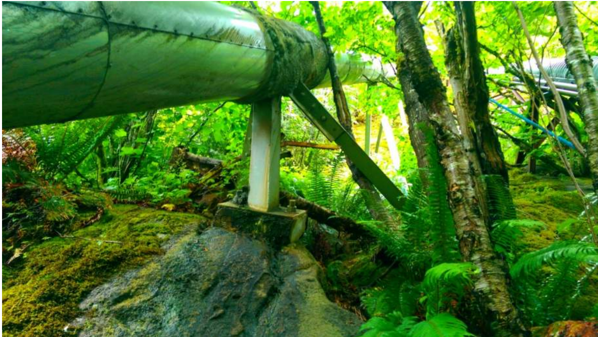
Photograph 14 South pipe bent.
