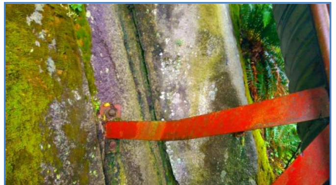
PHOTO 6: Bent support leg, likely from falling rocks
