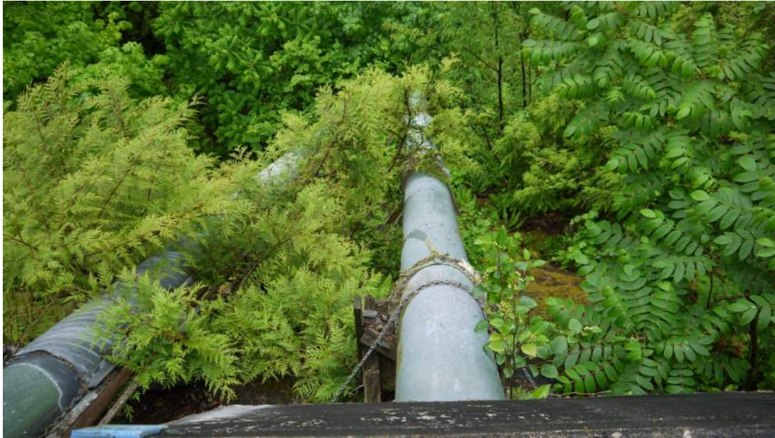
Photograph 1 Looking down pipe lines. North pipe is the left.
