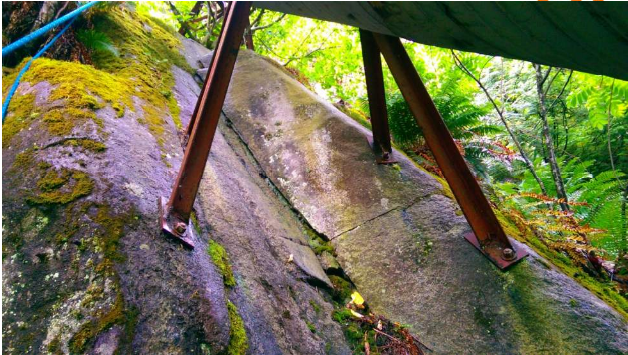
Photograph 15 North pipe bent – no diagonals are present.
