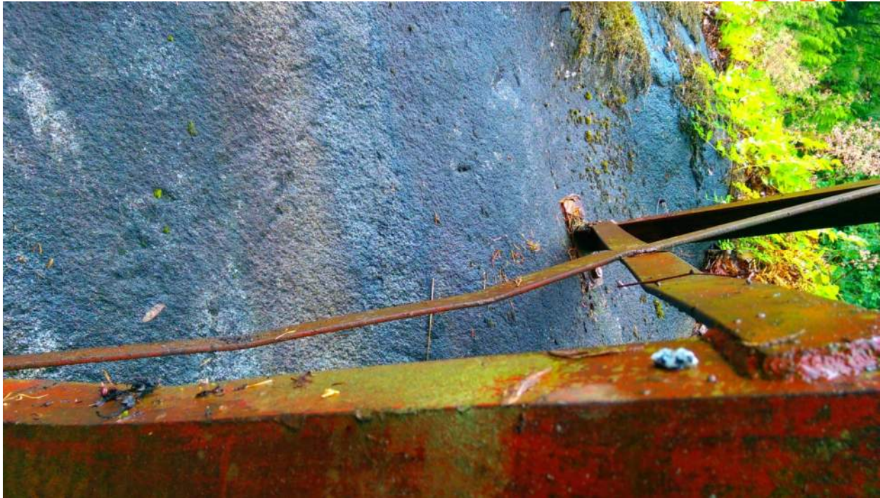
Photograph 9 Diagonal members damaged from falling debris.
