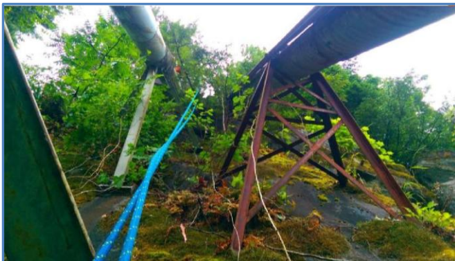
PHOTO 5: Typical supports, north pipe is on the right
