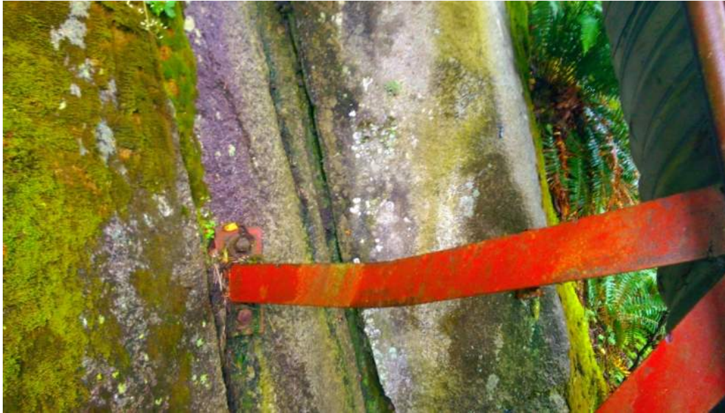
Photograph 13 Bent leg likely from falling rocks from above. Axial load capacity will be significantly reduced.
