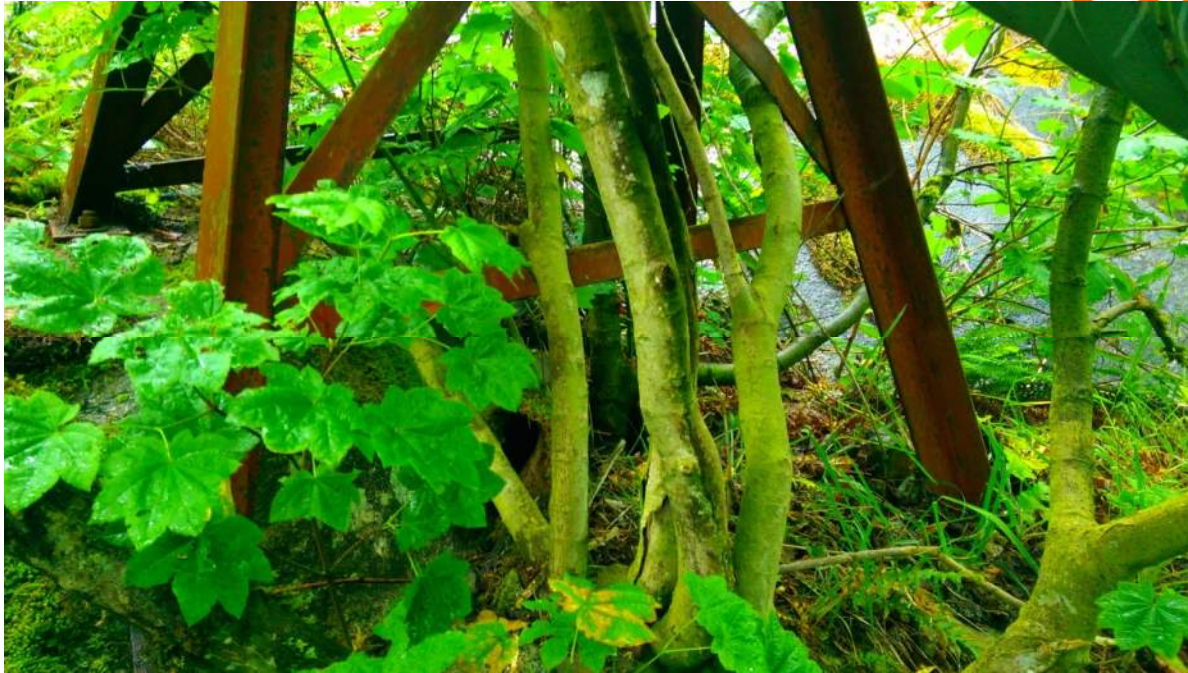
Photograph 11 Vegetation growth is deforming the bent diagonals. Baseplates should have all vegetation removed.
