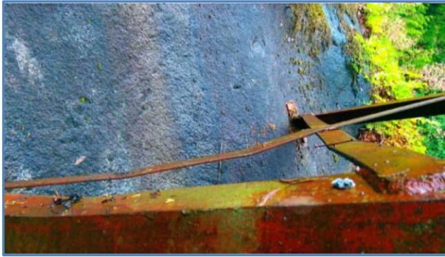
PHOTO 1: Diagonal members damaged
