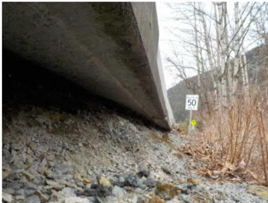
Photo 4: View of underside of road barrier showing extent of bearing material erosion
