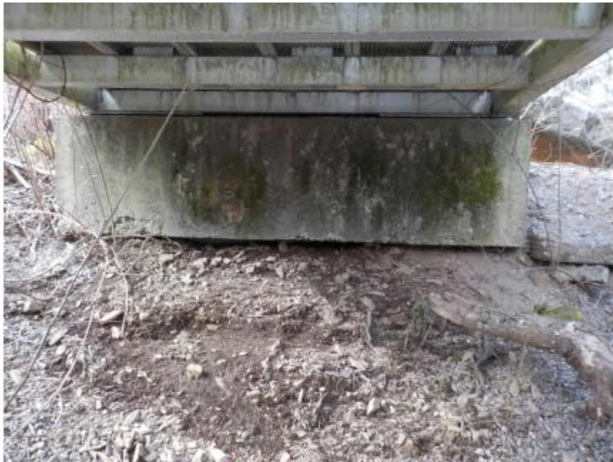
Photo 4: View of concrete abutment at west end. Light honeycombing at bottom left corner
