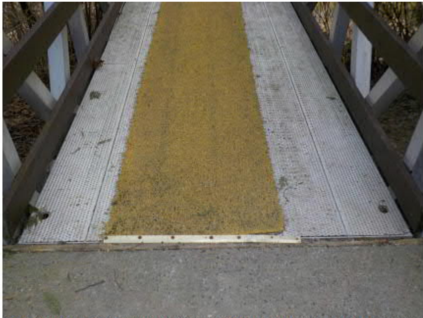
Photo 6: Caps missing at deck channels. Traction mat starting to loosen from support.
