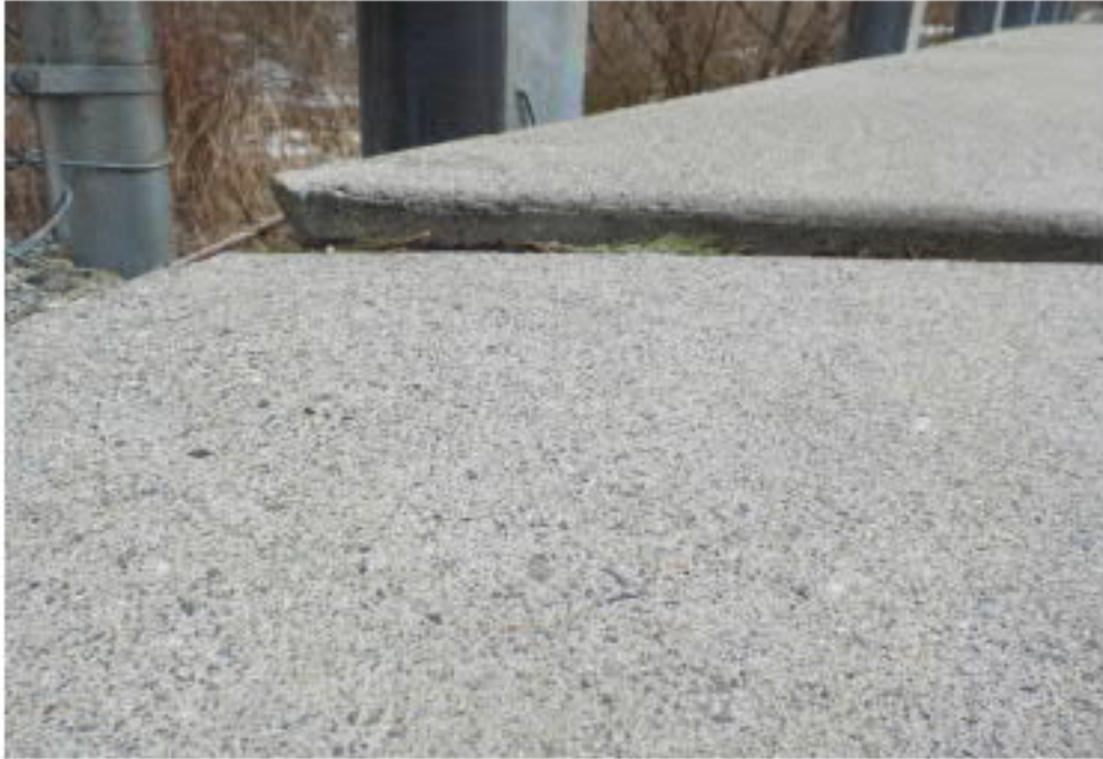
Photo 3: Differential settlement at sidewalk at bridge/approach interface
