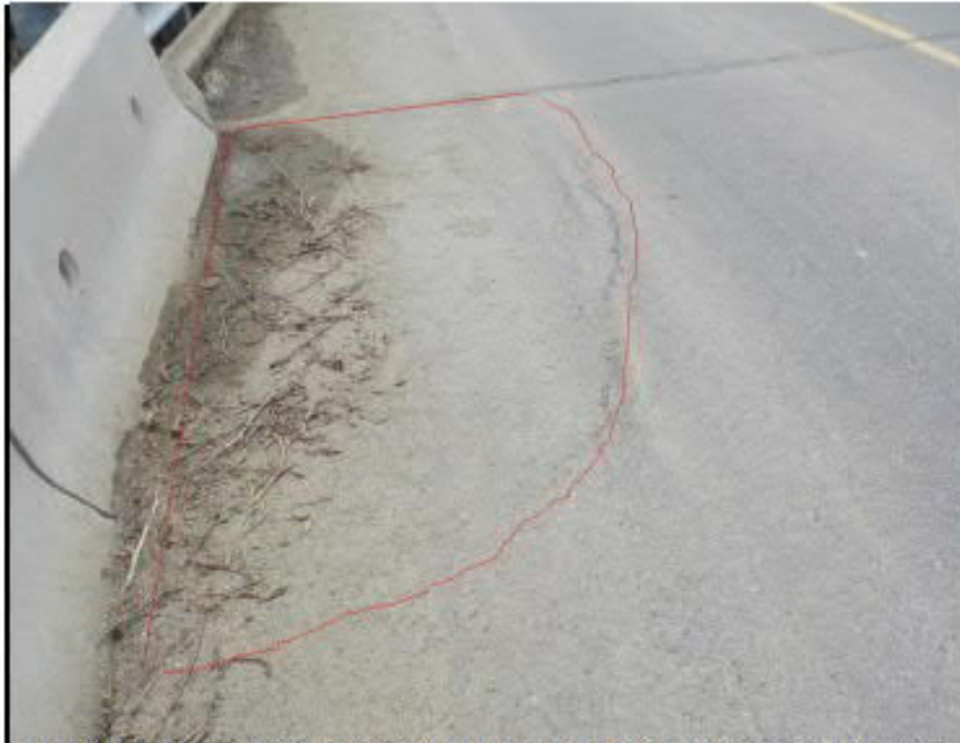
Photo 3: Localized settlement visible between asphalt crack and road barrier
