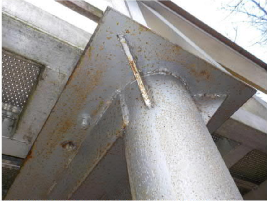
Photo 5: Minor general corrosion of protective coating at steel members
