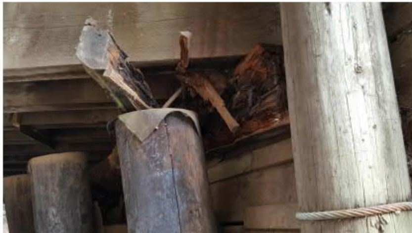
Photo 6: South abutment - note cap beam severely split and large gap between pile and ballast boards
