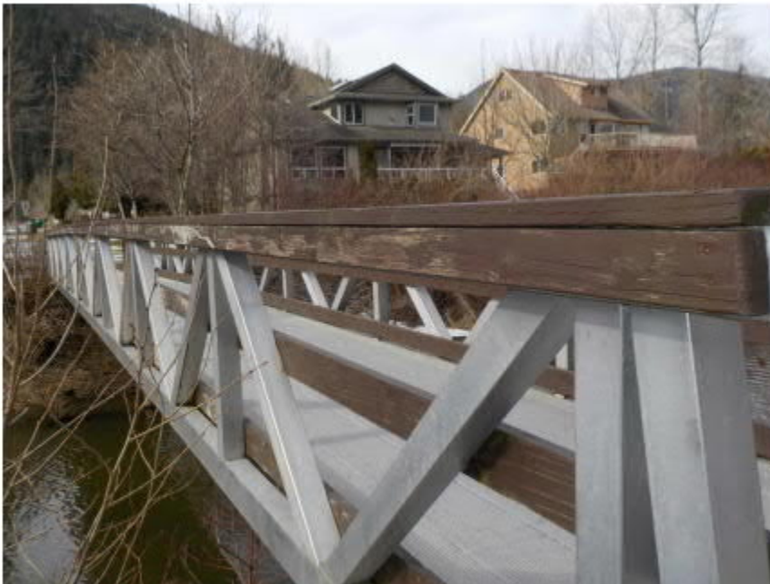
Photo 6: Side view of bridge. Full coating of paint was only applied on the inside face of the bridge.
