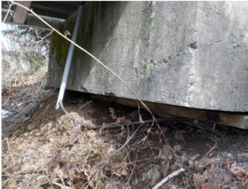
Photo 5: View of concrete abutment at east end. Erosion of abutment should be monitored.
