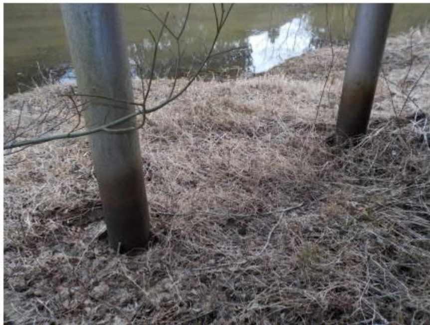
Photo 4: Protective coating corroded at the bottom portion of steel piles at pier support
