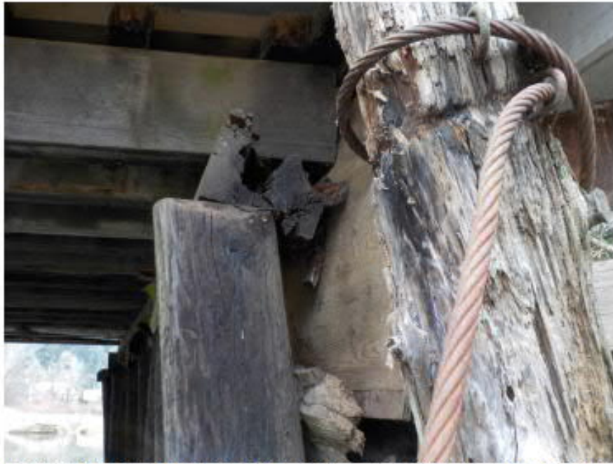
Photo 7: Cap beam and timber pile connection at north abutment. Note severe decay of cap beam.
