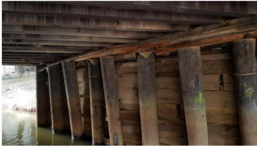
Photo 5: North abutment - note cap beam severely split and no longer bearing on top of piles
