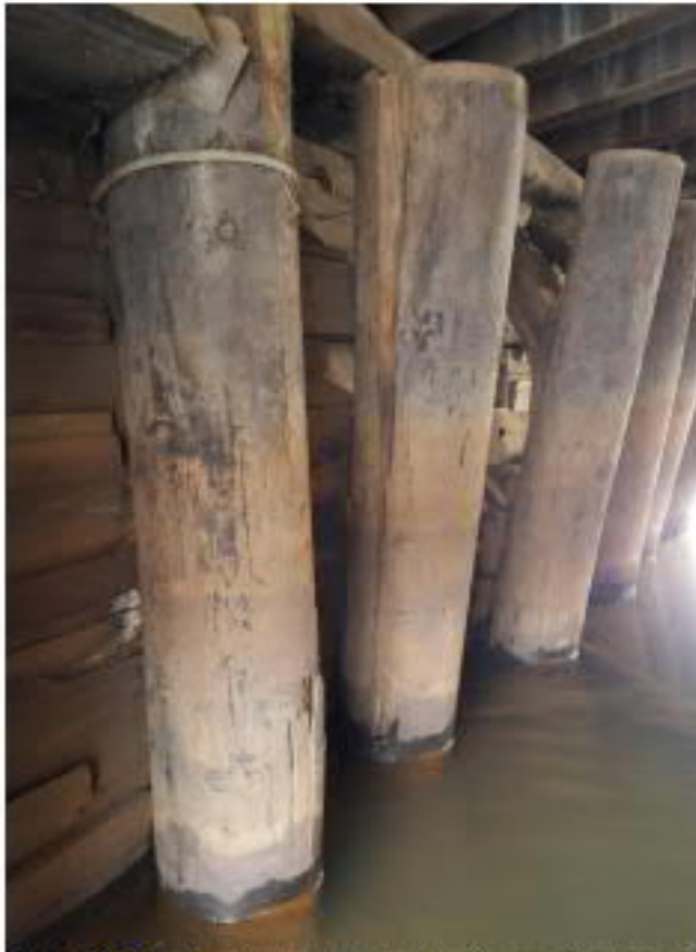
Photo 4: South abutment – Left pile cracked near bottom. Adjacent pile has severe split.
